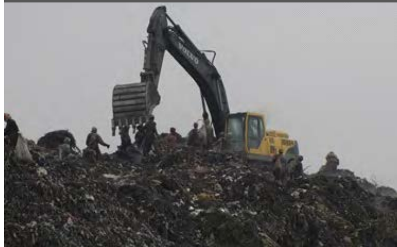
Exhibit 11.4. Informal Sector Workers in Close Proximity to an Excavator in Addis Ababa, Ethiopia
