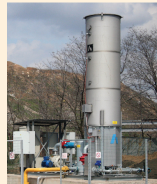
Landfill gas flare in operation at the Mariupol Landfill, Ukraine
