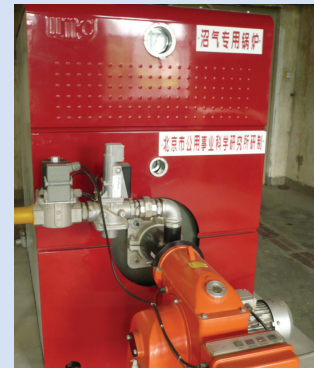
Landfill gas-fired boiler in operation at Gaoantun Landfill, China
