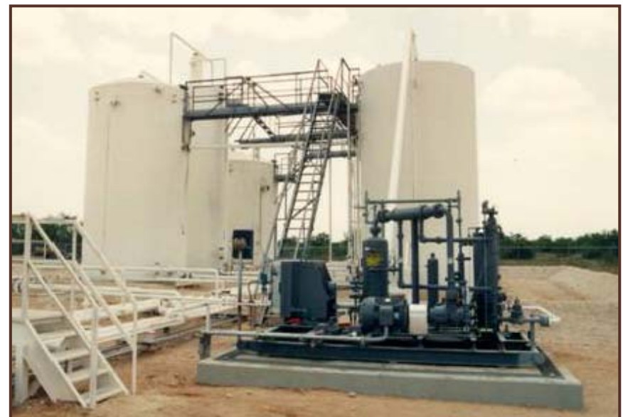
Source: Hy-Bon Engineering, VRU
