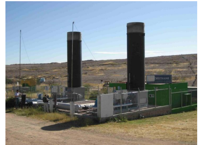
Aguascalientes – flare station & landfill
