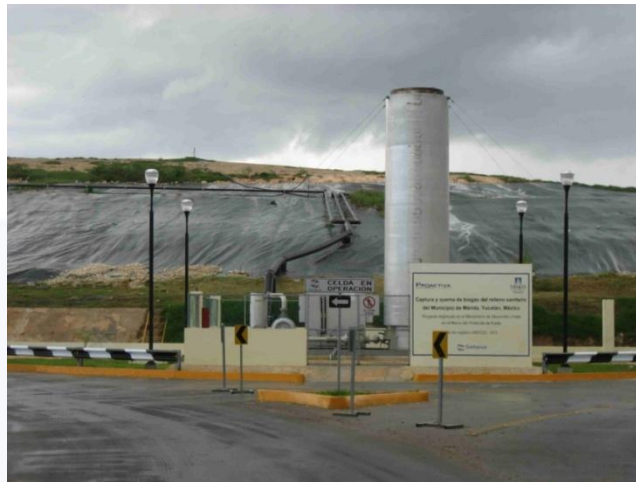
Merida – flare station & landfill
