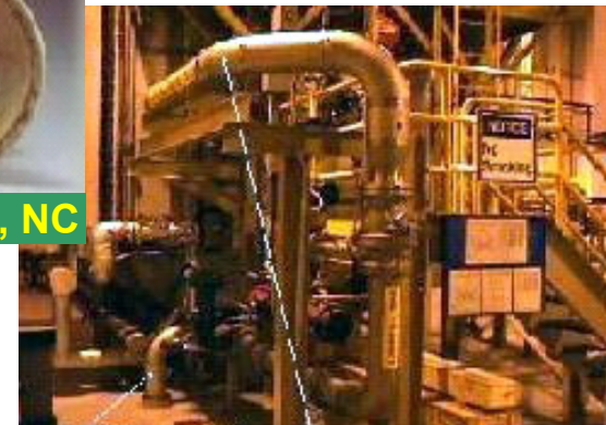
LFG-fired Boiler Ft. Wayne, IN
