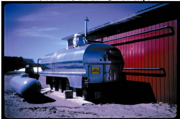
Hot Water Storage
