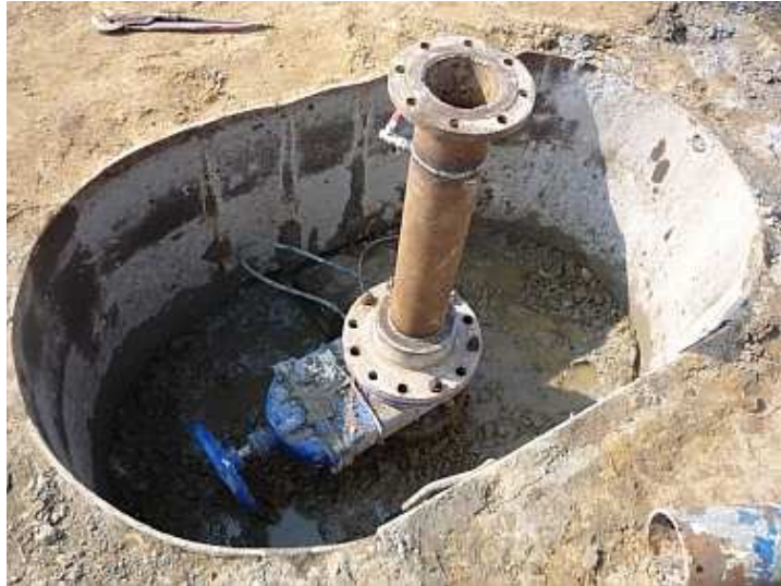
Figure 12. DN250 PN25 gate valve securing the borehole outlet
