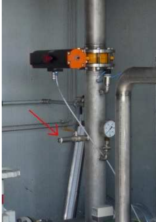
Figure 18. Gas sampling point
