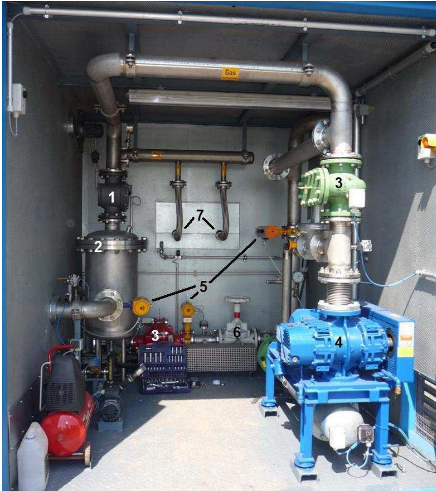
Figure 14. Engine room: 1 – filter, 2 – dehydrator, 3 – flame terminator, 4 – Roots' compressor, 5 – quick closing valve, 6 – manual valve, 7 – hoses to burners
