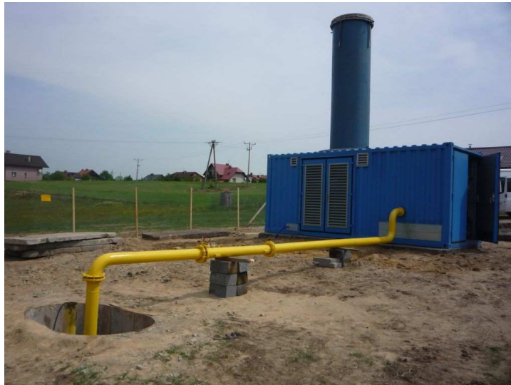
Figure 13. The borehole and the container station after completion of the drilling works
