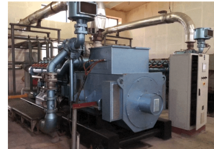
Gas-fired Generator – Working Mine, Pingdingshan, China
