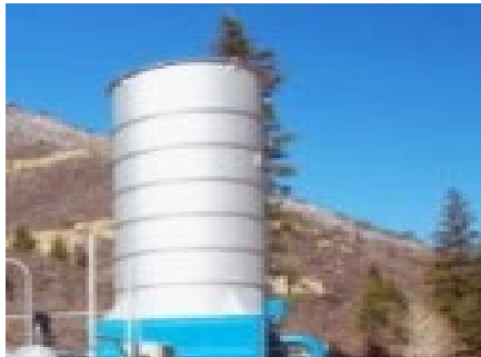
Abandoned Mine Methane Flare Colorado, USA
