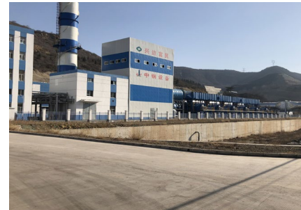
VAM destruction plant with 25 MW steam turbine to generate electricity Working Mine, Yangquan, Shanxi, China
