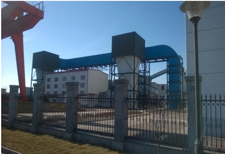
VAM Capture-hood at Top of VAM Shaft
