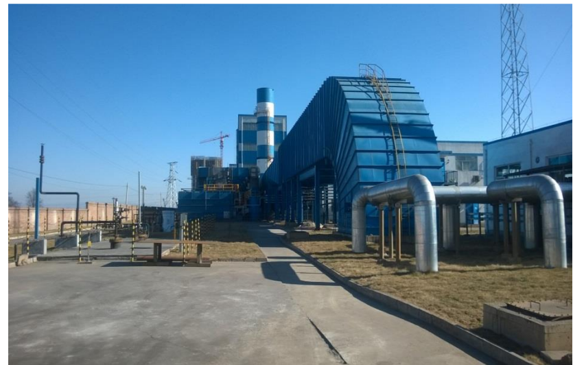
VAM Duct (1.08 Million M 3 /h)
