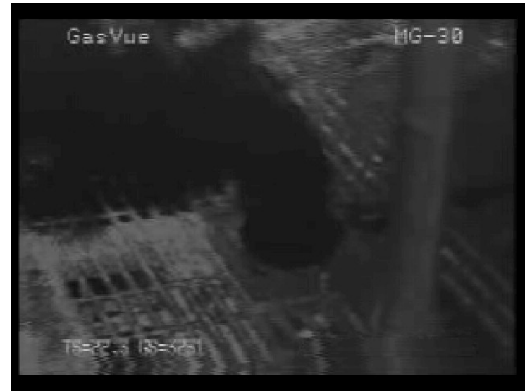
Infrared image from gas imaging device of open-end drain
