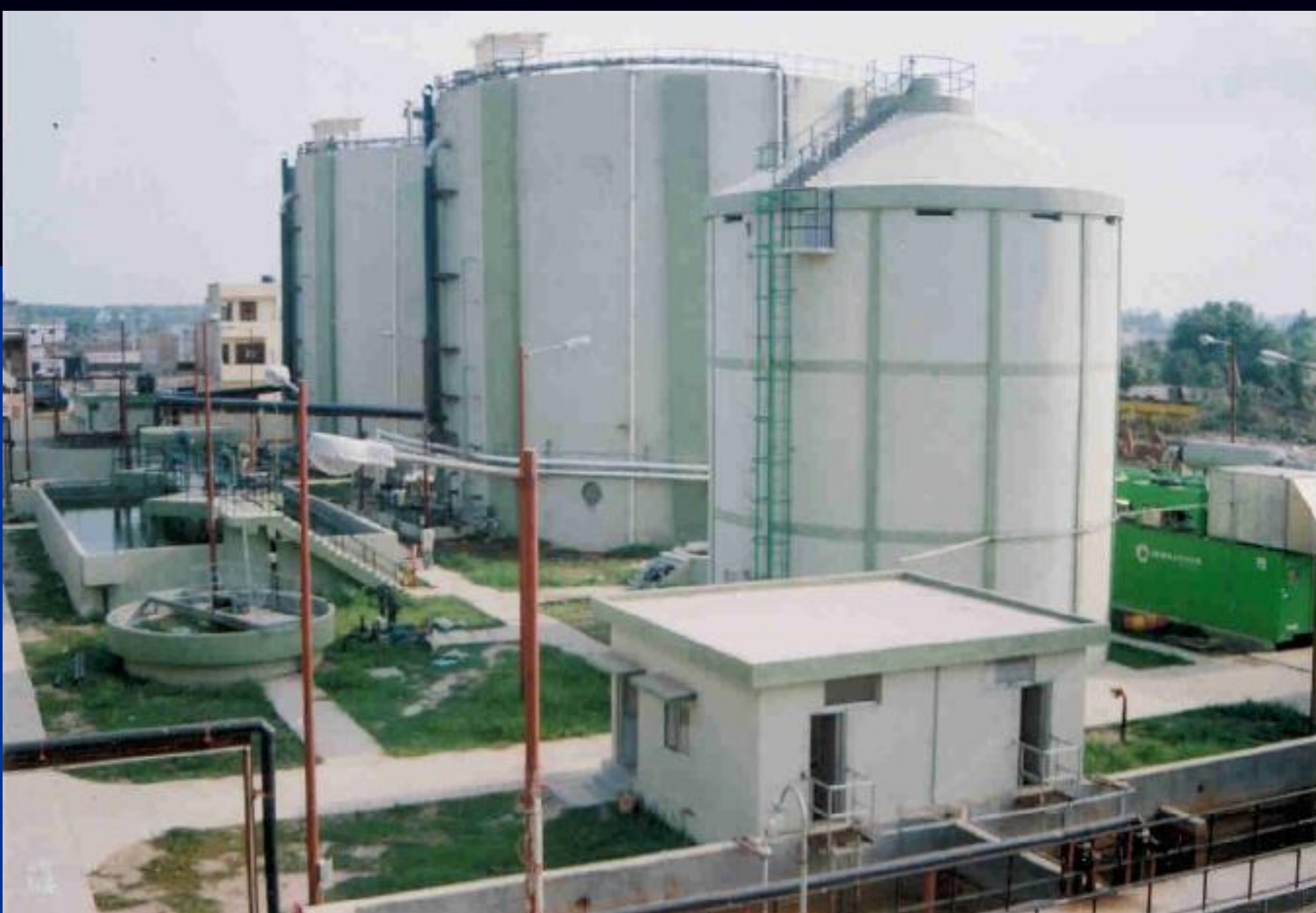
DIGESTER AND GAS HOLDER
