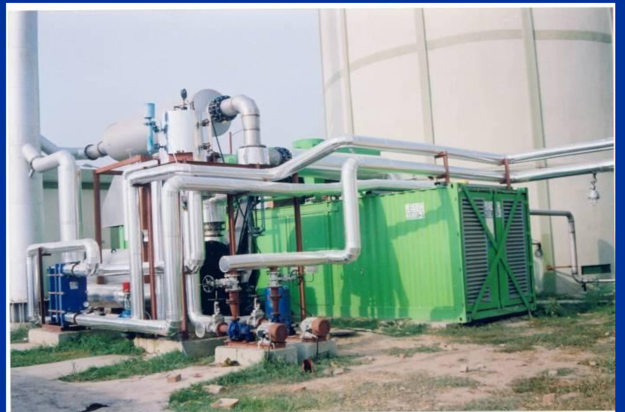
GAS ENGINE AND WASTE HEAT RECOVERY UNIT
