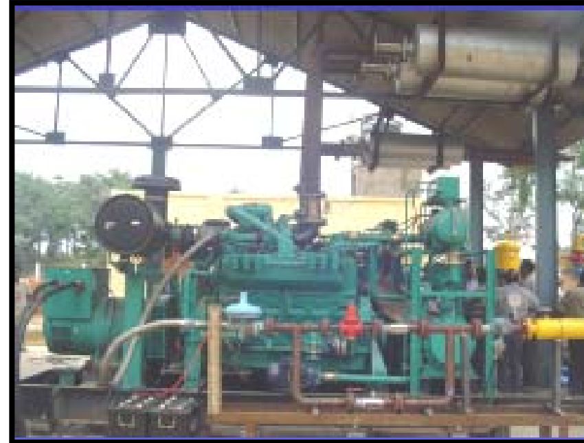
Gas based generator at Moonidih
