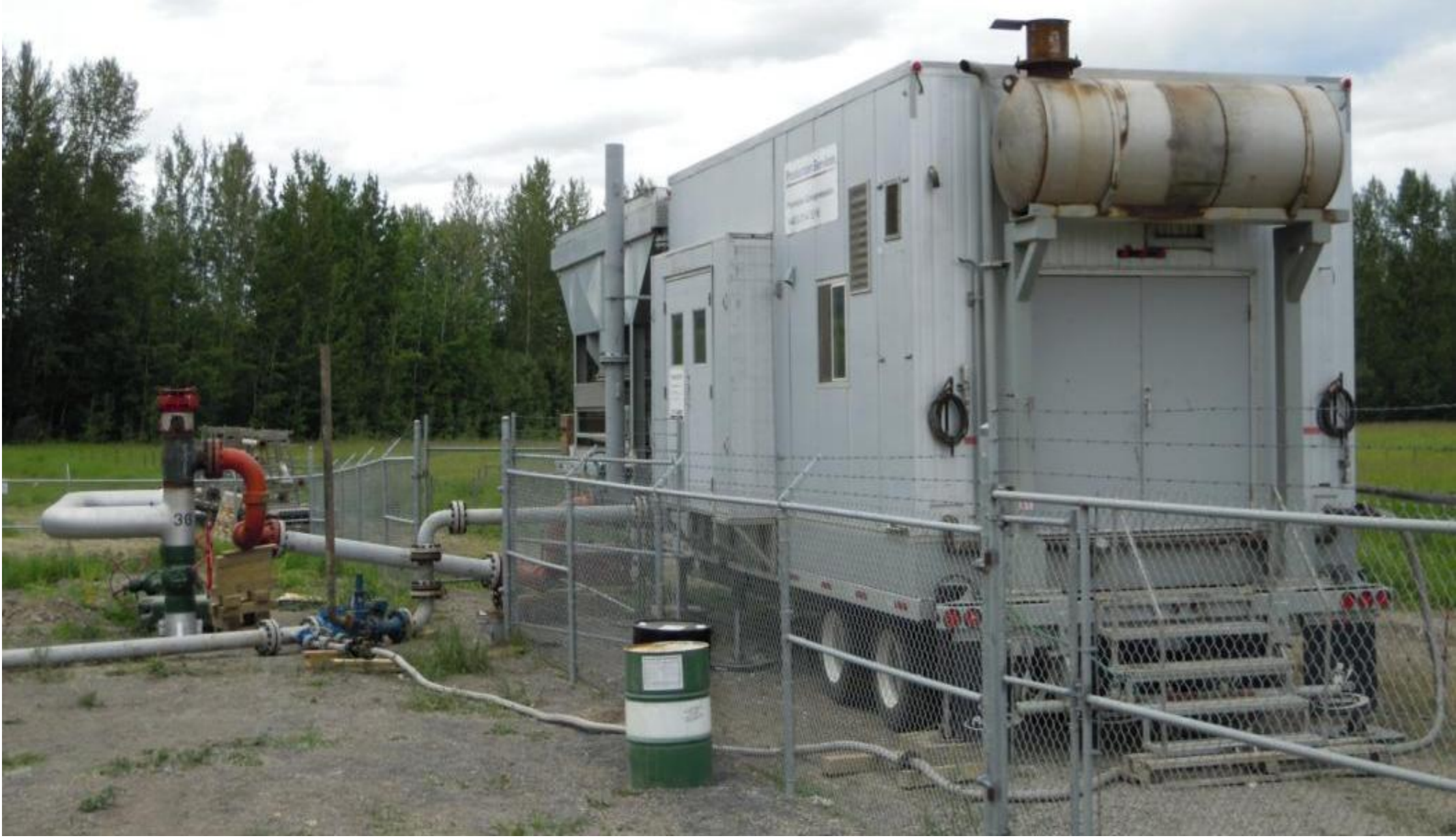
Mobile pump-down compressor in use on Spectra Energy's natural gas transmission pipeline to reduce venting of methane gas during maintenance activities.
