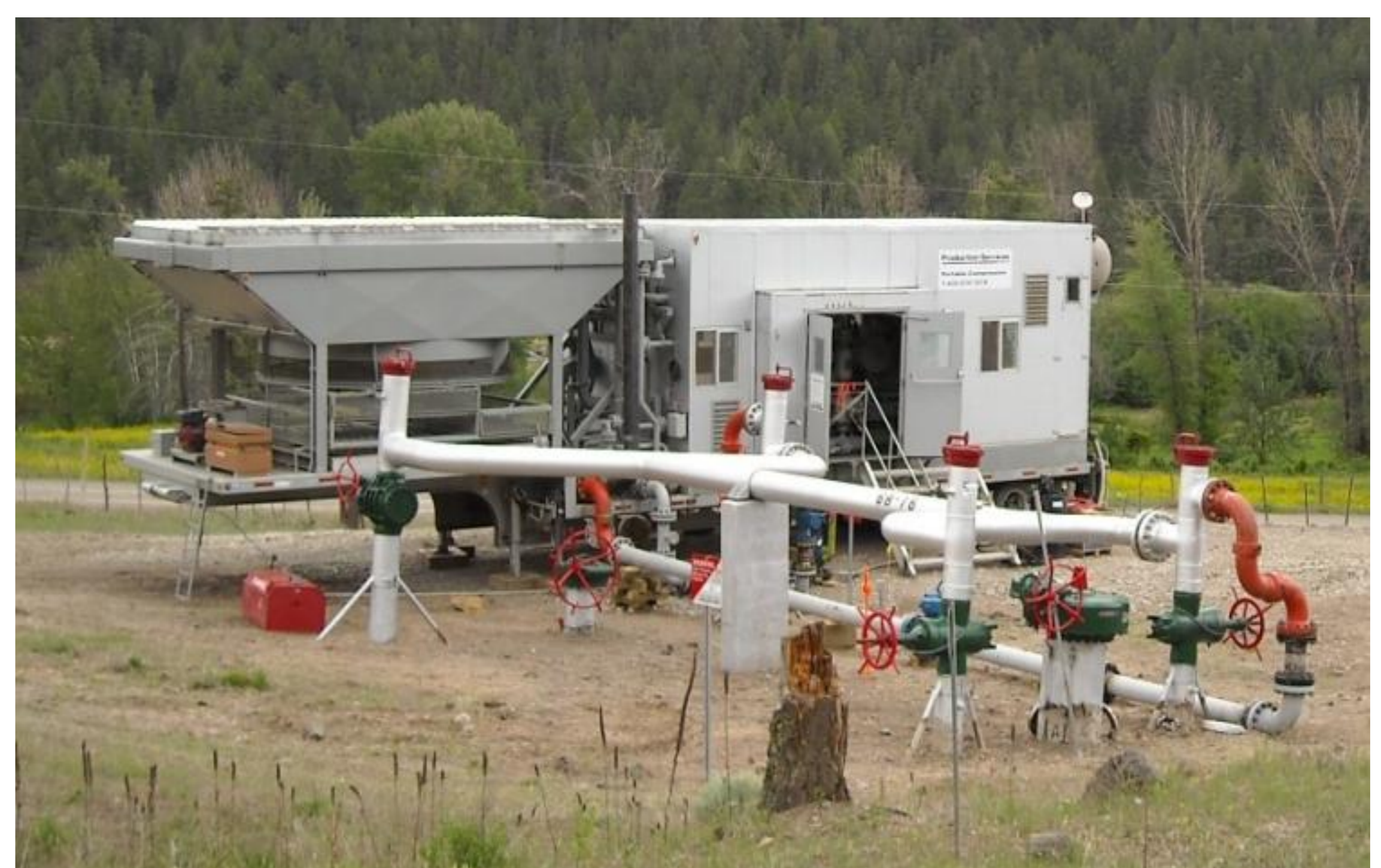
Mobile pump-down compressor in use on Spectra Energy's natural gas transmission pipeline to reduce venting of methane gas during maintenance activities.
