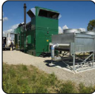
Toromont Power Systems installed this turnkey 1.6 MW digester-gas-fueled cogeneration system at the Woodward Avenue Wastewater Treatment Plant in Hamilton, Ont. It's powered by a Cat® G3520C gas engine configured for low-energy fuel.
