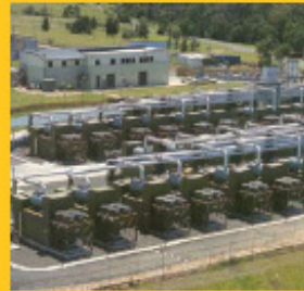
Aerial view of the Appin Power Station showing Caterpillar generator sets.
