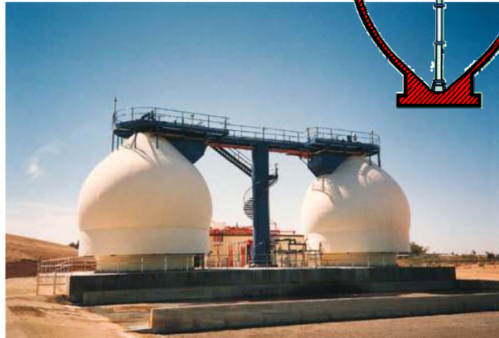
Egg-shaped digesters in Baltimore: designed to improve mixing and ease of solids removal (courtesy Sterling Fluid Systems)
