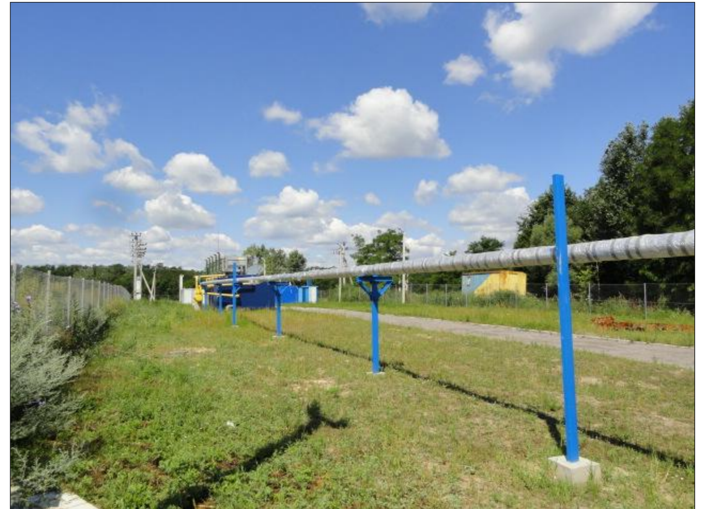
LFG transmission pipeline
