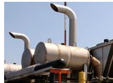
Landfill gas to energy
