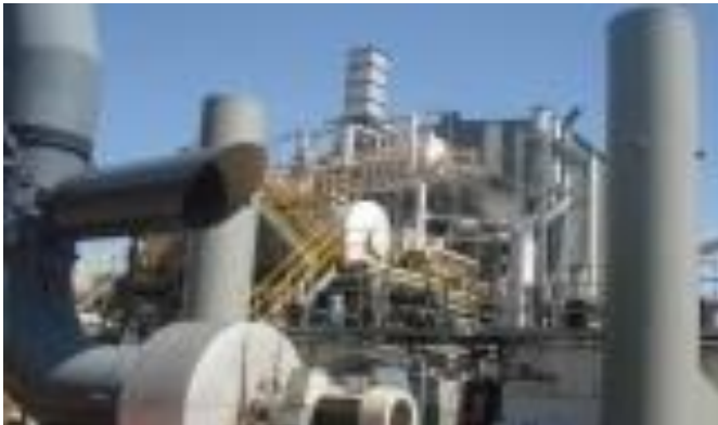
Coal mine methane capture
