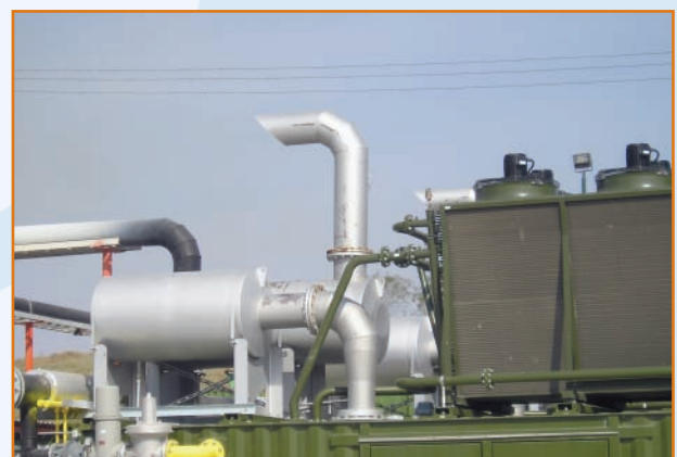
LFG engine generator at the Monterrey Landfill in Salinas Victoria.
