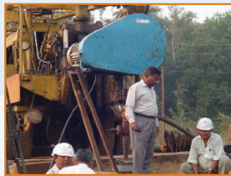
CMM pilot project at Moonidih Mine, India.
