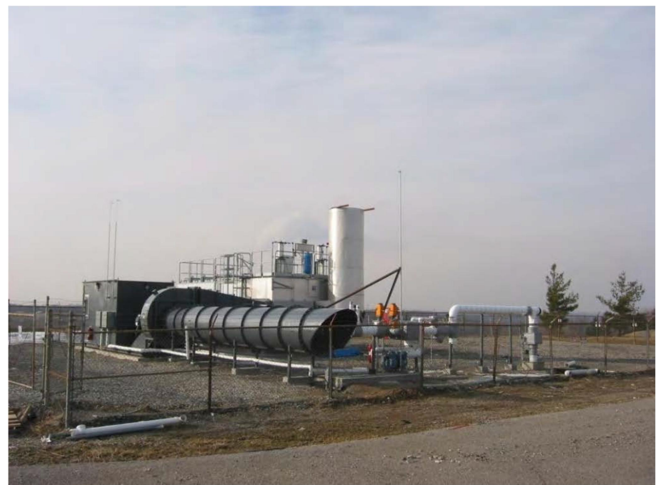
COMPLETED INSTALLATION AT WEST LIBERTY, WV
