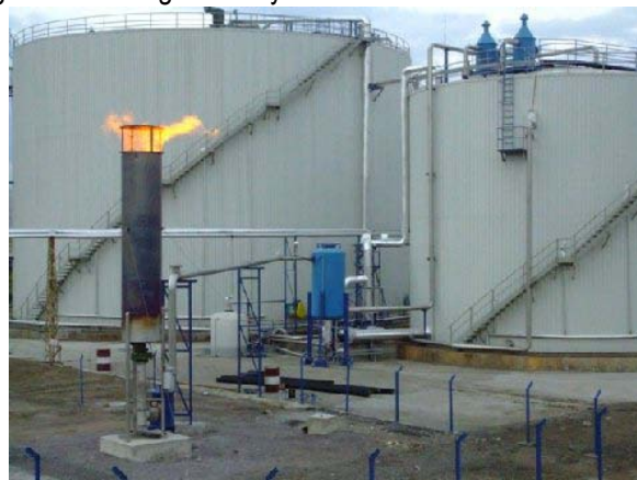
The anaerobic reactors and flare.
