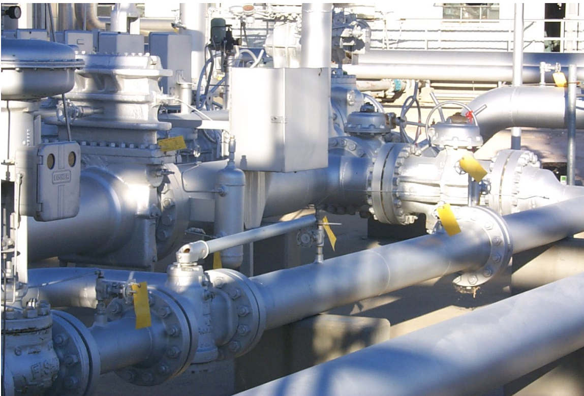
Figure 8: Photograph showing tagged fugitive equipment leaks at a gas processing facility
