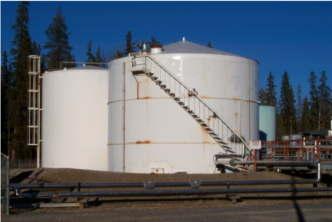
Figure 7: Photograph of hydrocarbon and produced water storage tanks at a production facility
